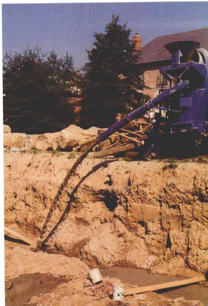
...or this. When concrete free falls more than about 5 ft., the aggregate can settle to the bottom. This seriously weakens the mix.
