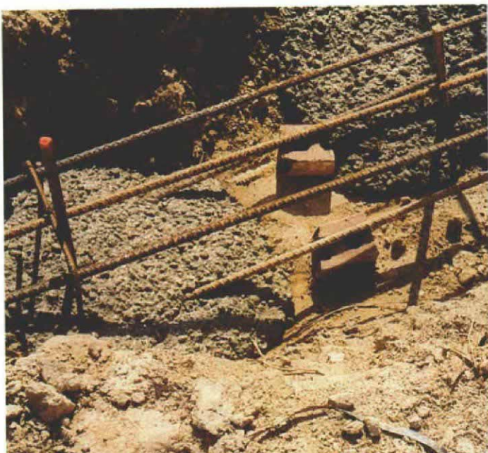
Don't do this. Elevating rebar on brick scraps is bad—but common—practice. Rebar should instead be supported on chairs.
