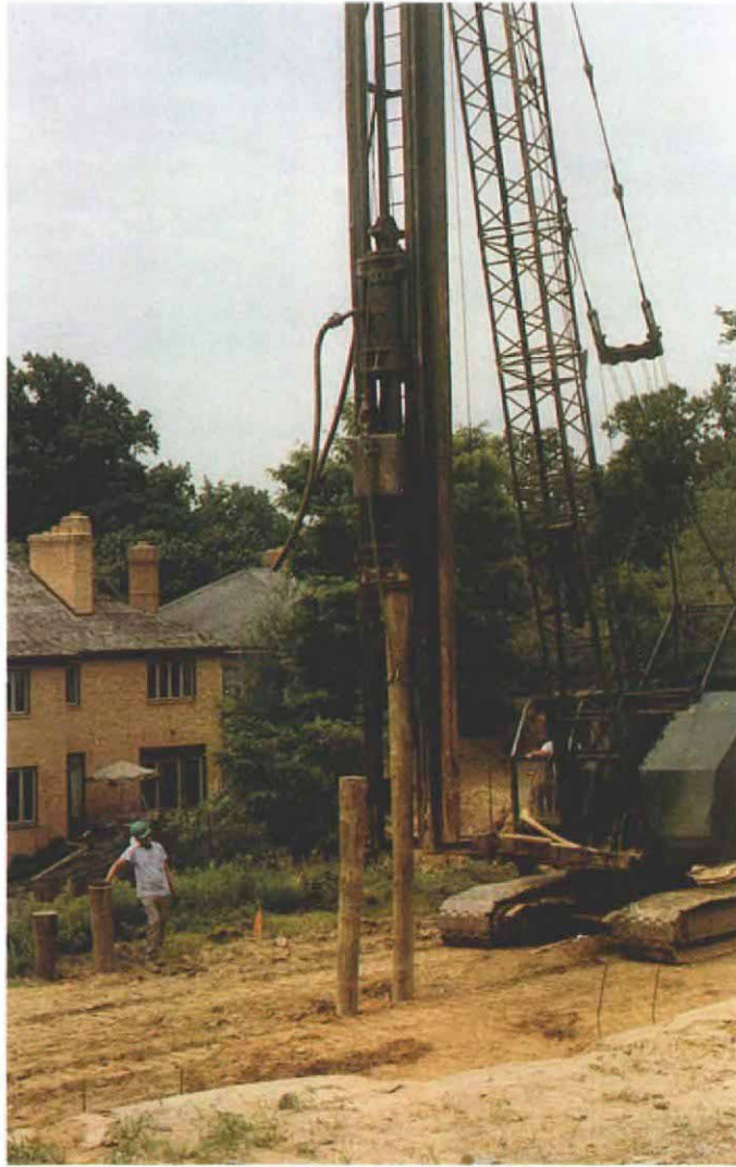
If I had a hammer. Wood piles are pounded in place with a pile driver. They're driven until they won't go any deeper (their "refusal depth"), even though the machine keeps hammering.
